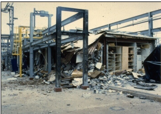
Explosion Damage to Control Room
