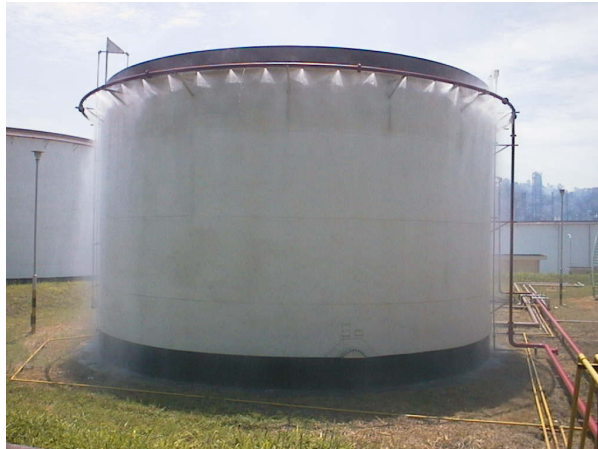
Storage Tank Deluge System
