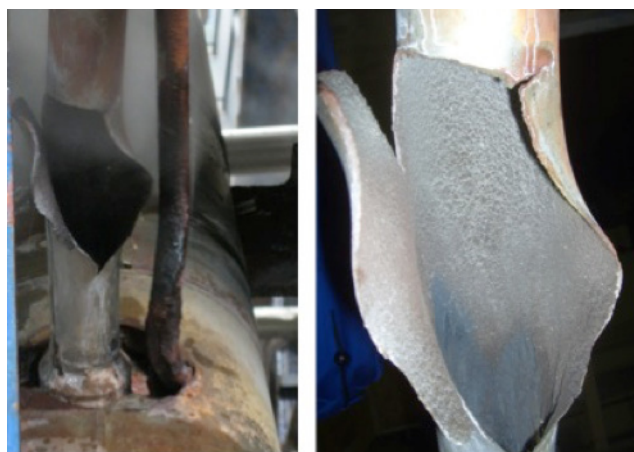
Figure 3. Rupture of a deadleg in a carbamate line.
