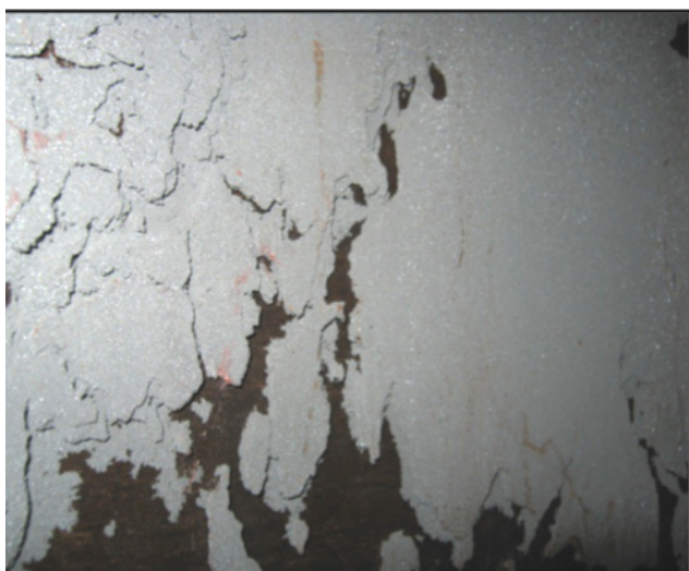
Figure 4. Carbamate condensate corrosion in type 316 UG plates.
