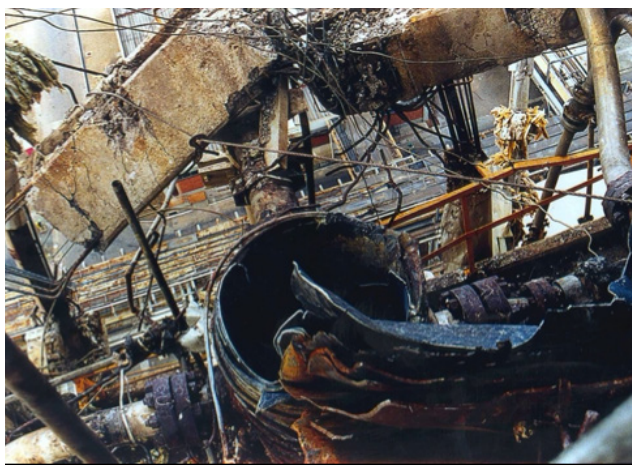
Figure 5. Carbamate corrosion failure of a high-pressure scrubber.
