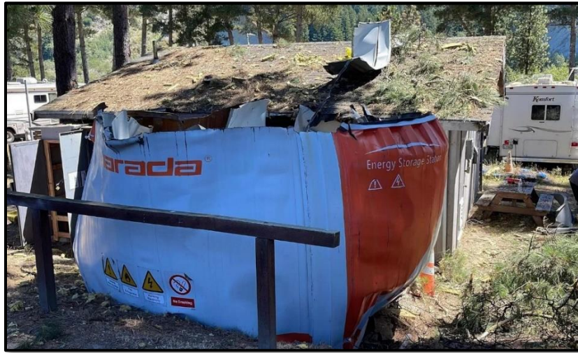
Figure 2 – Lead acid battery explosion (likely due to hydrogen) 2
