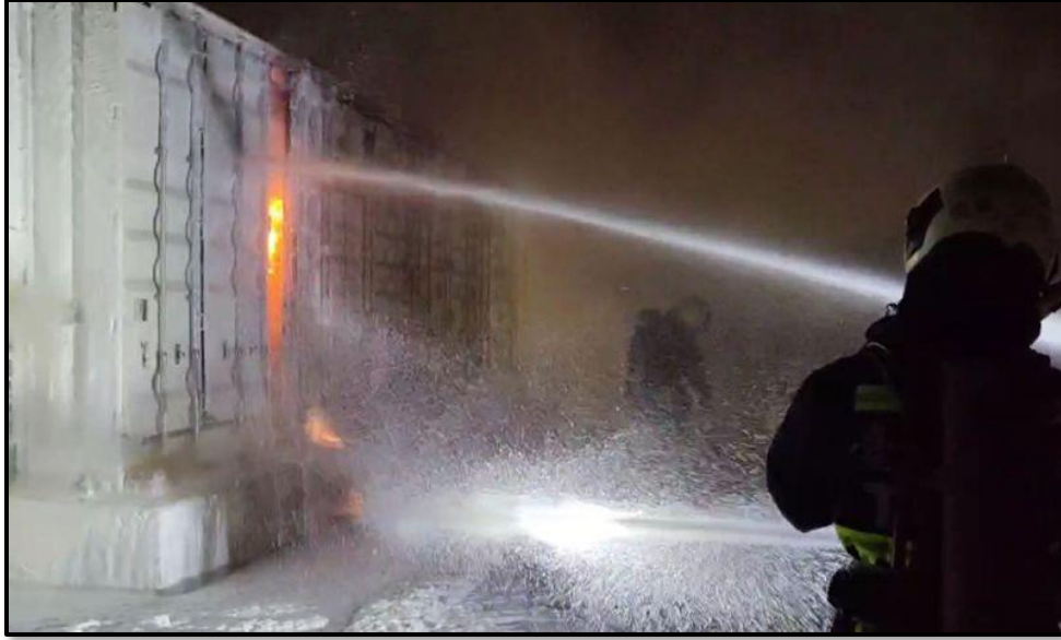
Figure 5: Reported LPF Battery fire at in Longjing District, Taichung City, Taiwan, July 2023 5
